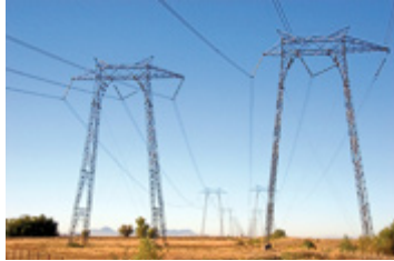
Electric transmission lines near Richvale, California. DAVID R. FRAZIER/DANITA DELIMONT AGENCY /DRR.NET
